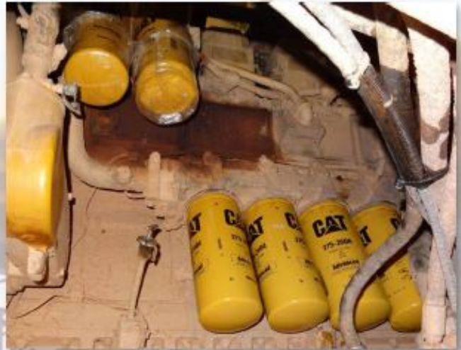
Engine oil: four CAT 275-2604 filters (bottom).
